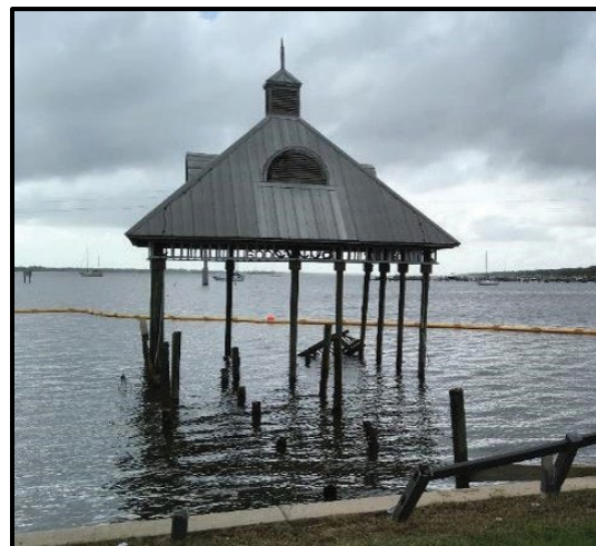
2017 Hurricane Irma Damage
